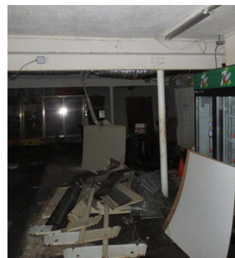
photo: store interior. Exposed cabling is not permitted by NEC. Lighting is fluorescent.
