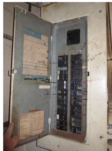
photo: main panel in existing store space. This panel is obsolete & beyond expected service life.
