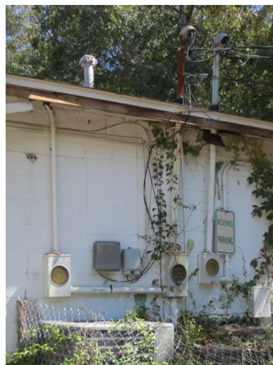
photo: service/meter at west end of building. Additional service is at the east end.
